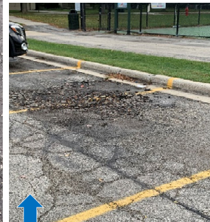
Example of parking lot failure
